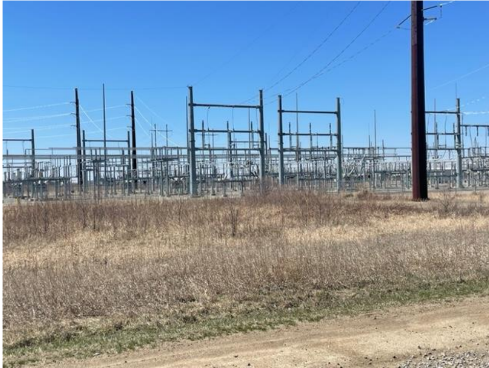
The Marshalltown Substation on the east side of Marshalltown, Iowa.
