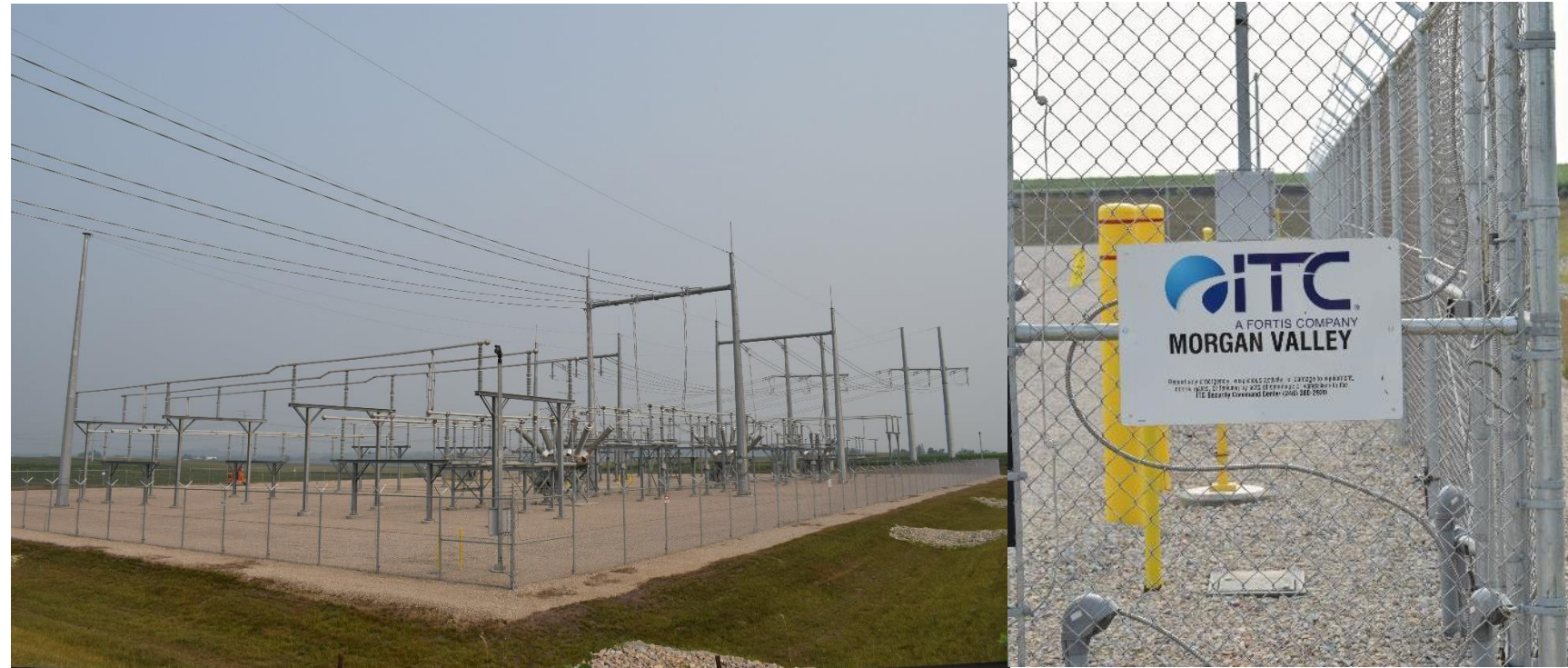
Morgan Valley Substation near Fairfax, Iowa
