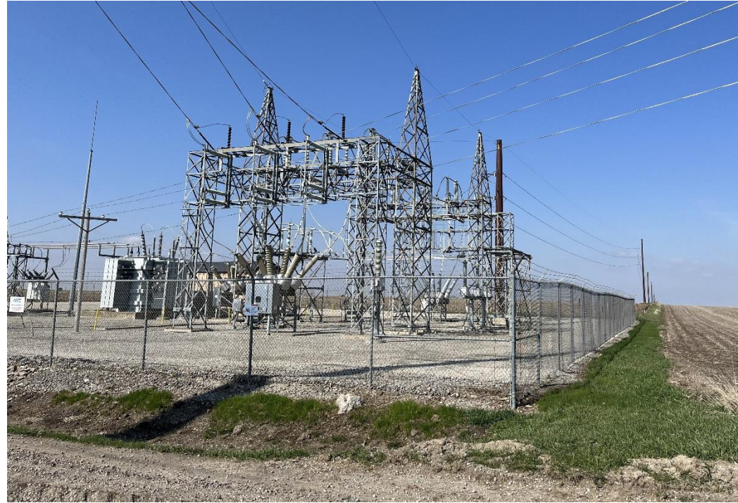
The Belle Plaine Junction Substation north of Belle Plaine, Iowa.
